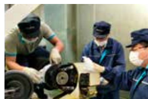
WCM Labeling & Cleaning - 735 labels were applied and nearly 90 areas were identified and cleaned.
